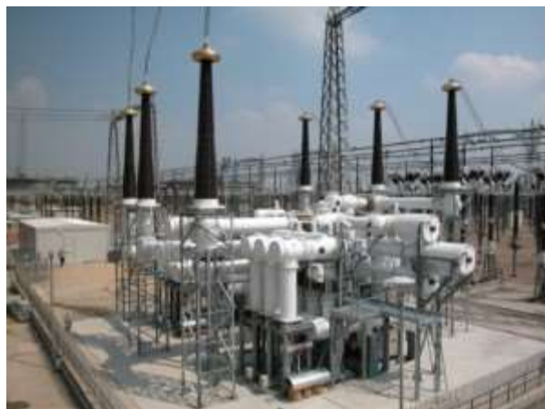
Figure 268: A high voltage breaker (Image Dingy under the CC-BY-SA 3.0 license)
