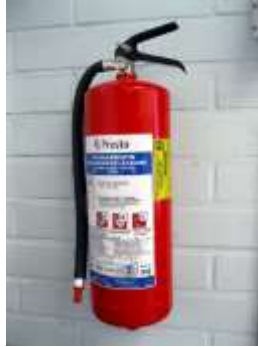
Figure 345: Fire Extinguisher on a Wall (Image Santeri Viinamäki under the CC-BY-SA 4.0 license)
