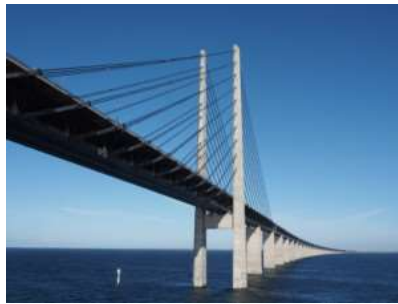
Figure 124: Öresund Bridge in direction to Kopenhagen (Image Hajotthu under the CC-BY-SA 4.0 license)
